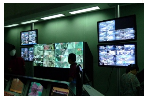
NUUO CMS Matrix | At RapidKL Central Control Room
